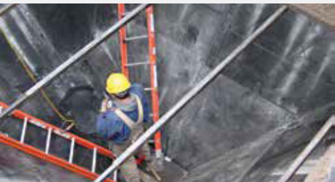
Coal Receiving Hopper Liner
